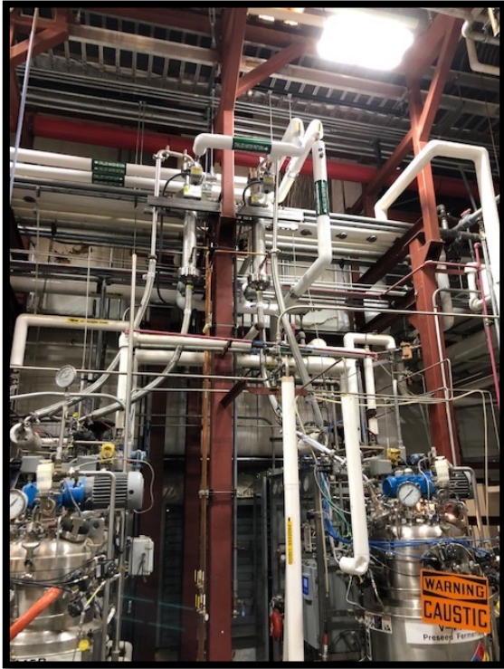
Knockback condensers installed on the two 160-L bioreactors
