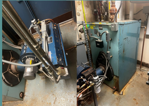
Pictured Above: An example of aging critical infrastructure in the school. Two low efficiency heating oil boilers installed in 1982. NCS D has not been able to source parts for years outside of eBay. One boiler is currently inoperational.
