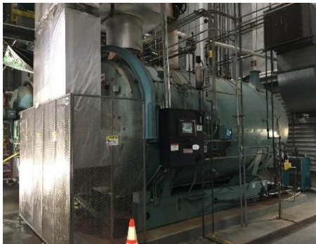
Heat Recovery Steam Generator (HRSG): Source – PepsiCo
