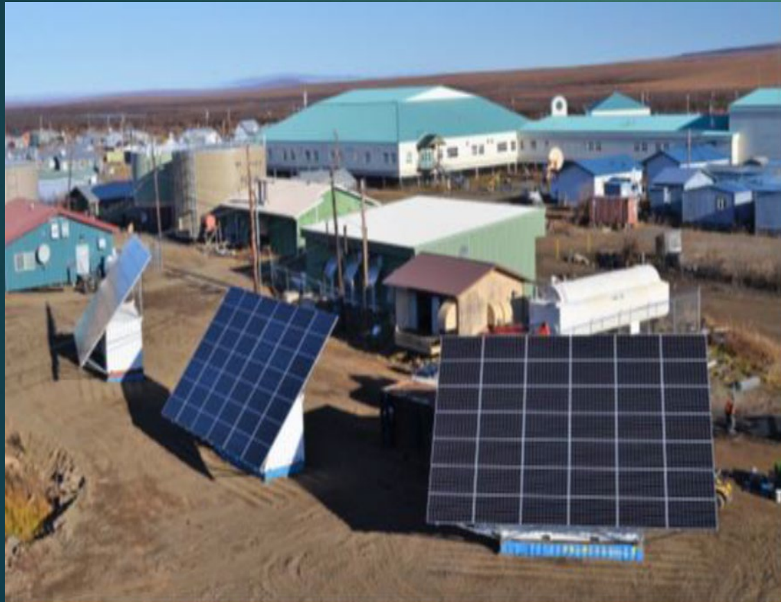
Buckland Solar arrays, Courtesy NANA
