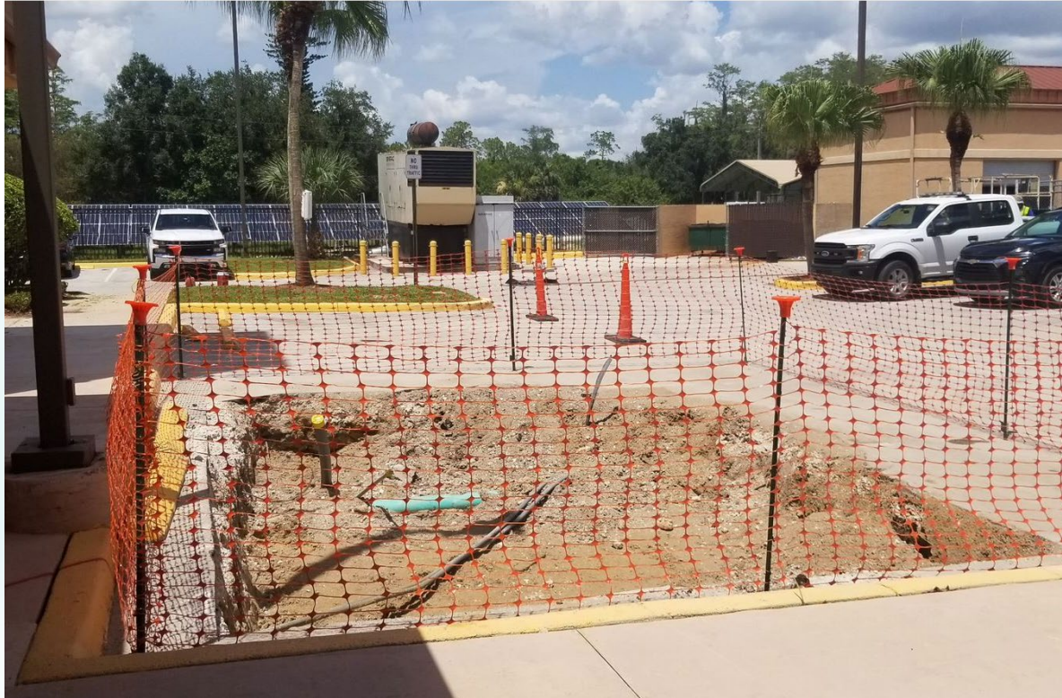
Unmarked sanitary sewer line conflict
