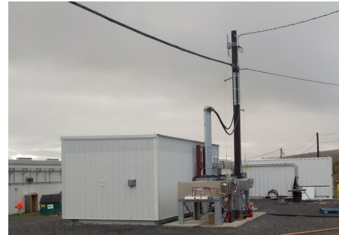
New Data and Communications Center
