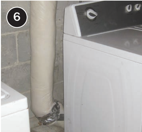
Duct in unconditioned space is insulated.
