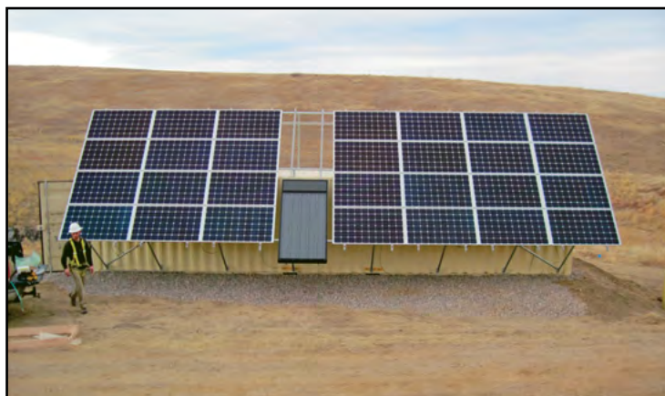
Solar installation at Rocky Flats Site, Colorado.
