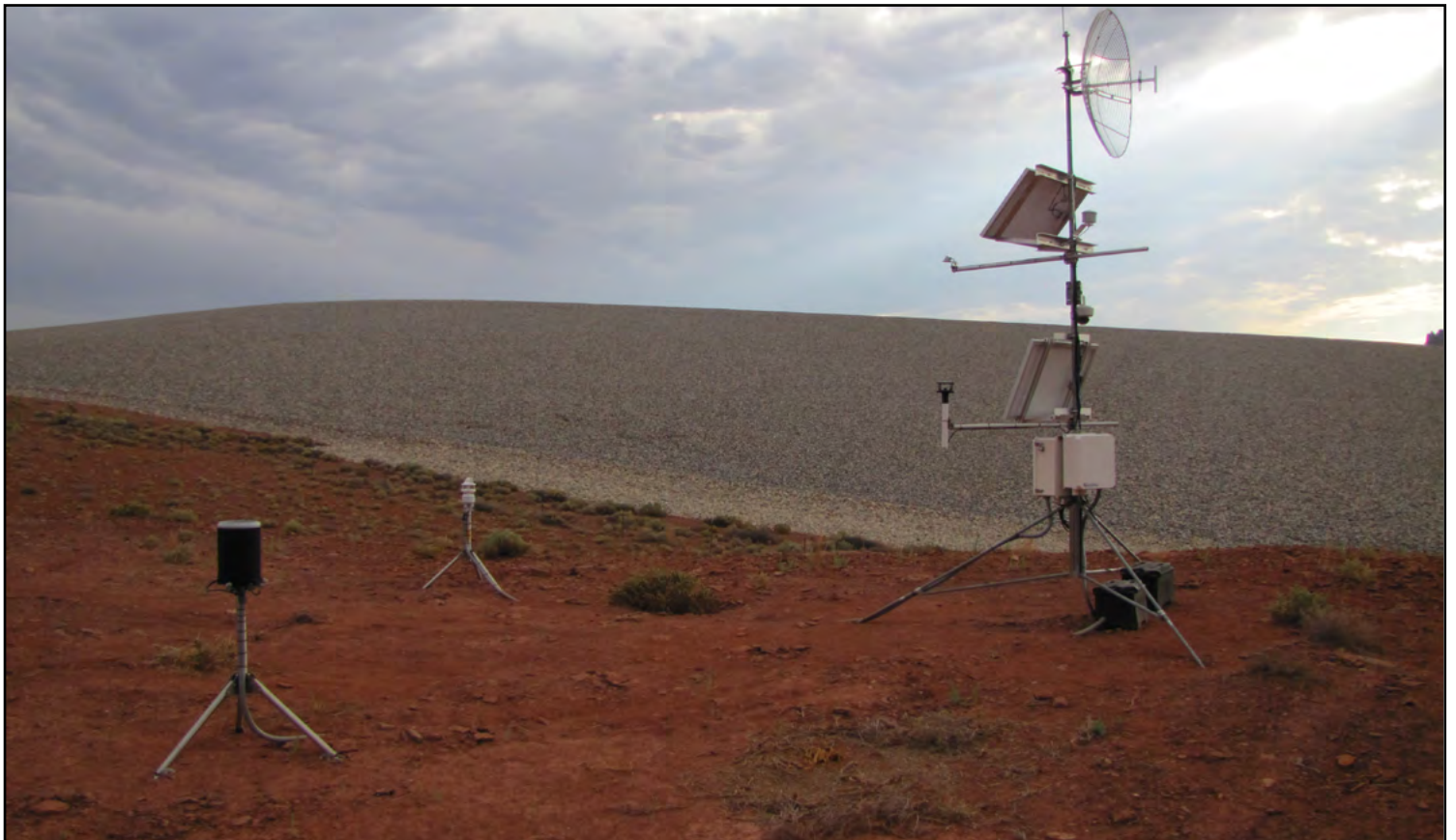
A large number of intense precipitation events between 2009 and 2018 likely contributed to water erosion below the rock cover on the disposal cell at the Mexican Hat, Utah, Site. LM is undertaking repairs to the cell to protect against erosion under the surface.
