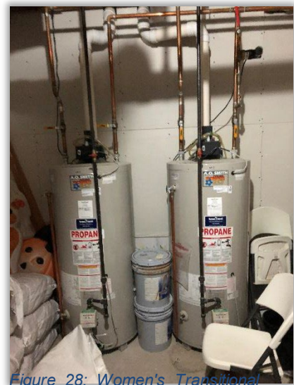
Figure 28: Women's Transitional Living Water Heaters
