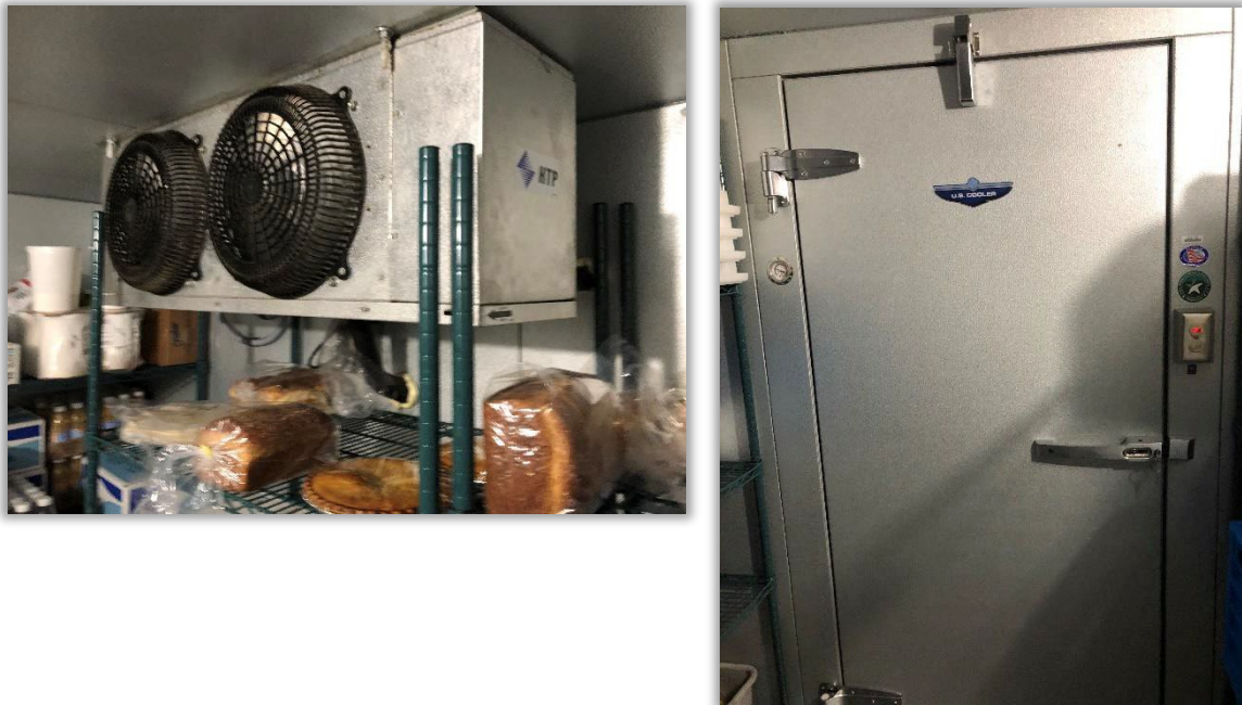
Figure 25: Caring Place Walk-in Cooler Shaded Pole Fan (left) and Walk-in Freezer Door (right)
