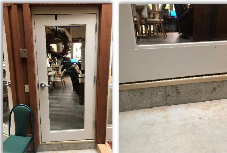
Figure 22: Door to Center Room Housing the Tree (left) and its lack of weatherstripping (right)
