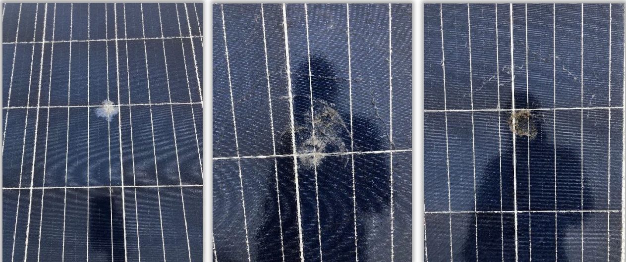
Figure 30: Women's Transitional Living Damaged Solar
