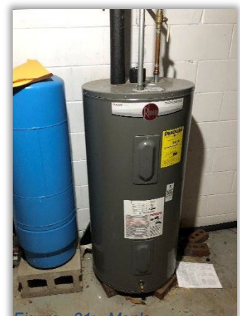
Figure 31: Men's Transitional Living Water Heater
