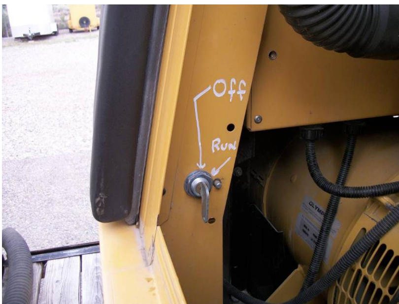
Figure 2. Battery Isolation Switch
