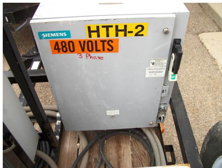
Figure 4. Typical Disconnect Switch
