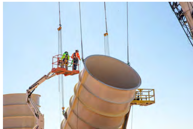
Workers attach guiding tag lines to ductwork before lowering it into a channel adjacent to the utility shaft at WIPP.
