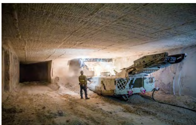
A continuous miner machine in WIPP’s underground chews through a final section of salt to finish the preliminary rough cut of Panel 8.
