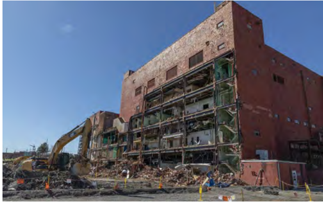
Crews take down the six-story Building 9207 at the former Biology Complex at Y-12. The 1940s-era building spanned 255,000 square feet and was listed as a high-risk facility.
