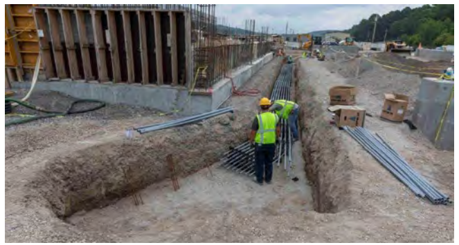
View of construction progressing at the Mercury Treatment Facility. When operational in 2025, it will be able to treat up to 3,000 gallons per minute.
