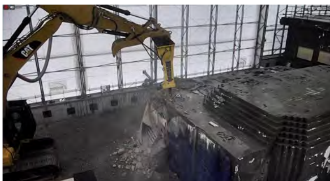
Crews remove the former Radiological Development Lab’s West Cell Bank at ORNL. Crews built a protective cover over the structure to ensure a safe teardown of the high-risk contaminated structure.
