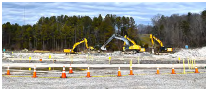
Heavy equipment tears up the largest remaining slab at ETPP, which was where the former Centrifuge Complex once stood.
