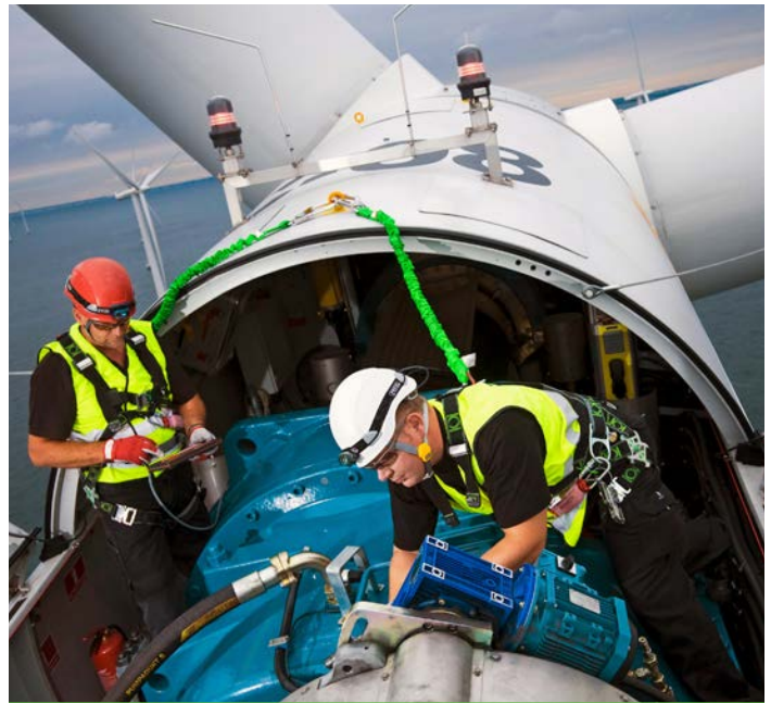
Photo from Siemens AG, NREL 19687
