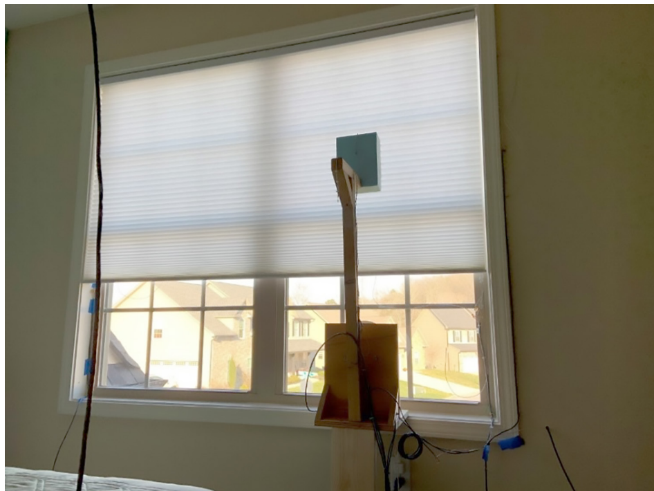
Cellular shade installed at ORNL's Yarnell Station house.
