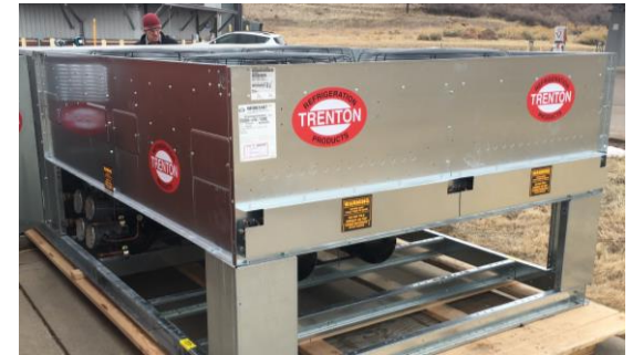
60 horsepower chiller at NREL's site
