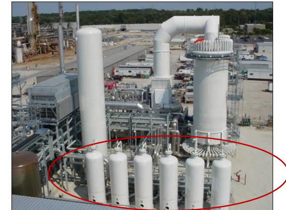
PSA Purification System
