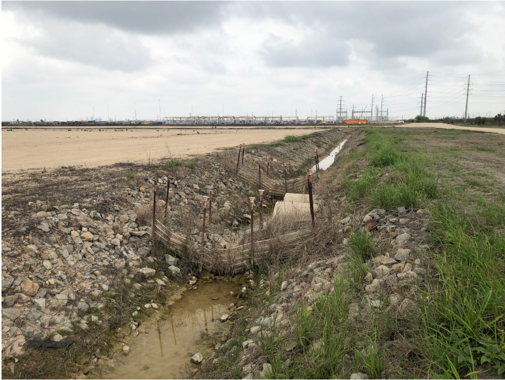
Water quality best management practice installed at 110-acre Port Laydown. Photo taken April 13, 2021.
