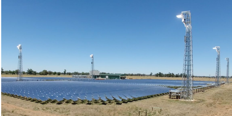
Figure 2. Vast Solar's 5-MW th Jemalong pilot plant has derisked sodium handling in preparation for their proposed Mt. Isa project. Vast's commercial system will operate at sodium temperatures up to about 600°C and employ thermal energy storage with nitrate solar salt. Photo: Vast Solar
