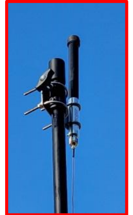
Road Side Unit (RSU)
