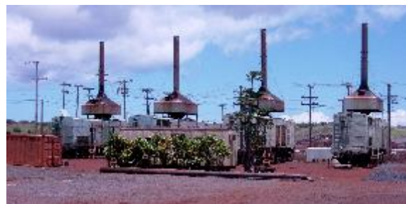
(6) 1.0 MW EMD Diesel Generators (2) 2.2 MW Caterpillar Diesel
