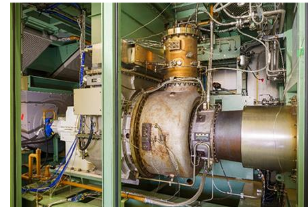
IHI 70% liquid NH 3 cofiring 2MW-class gas turbine, 2020
