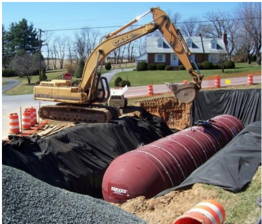
30,000 gallon underground tank Capital cost ~$100K
