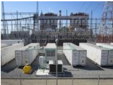
5 MWh A123 battery in Chile Capital cost $50,000 - 100,000K
