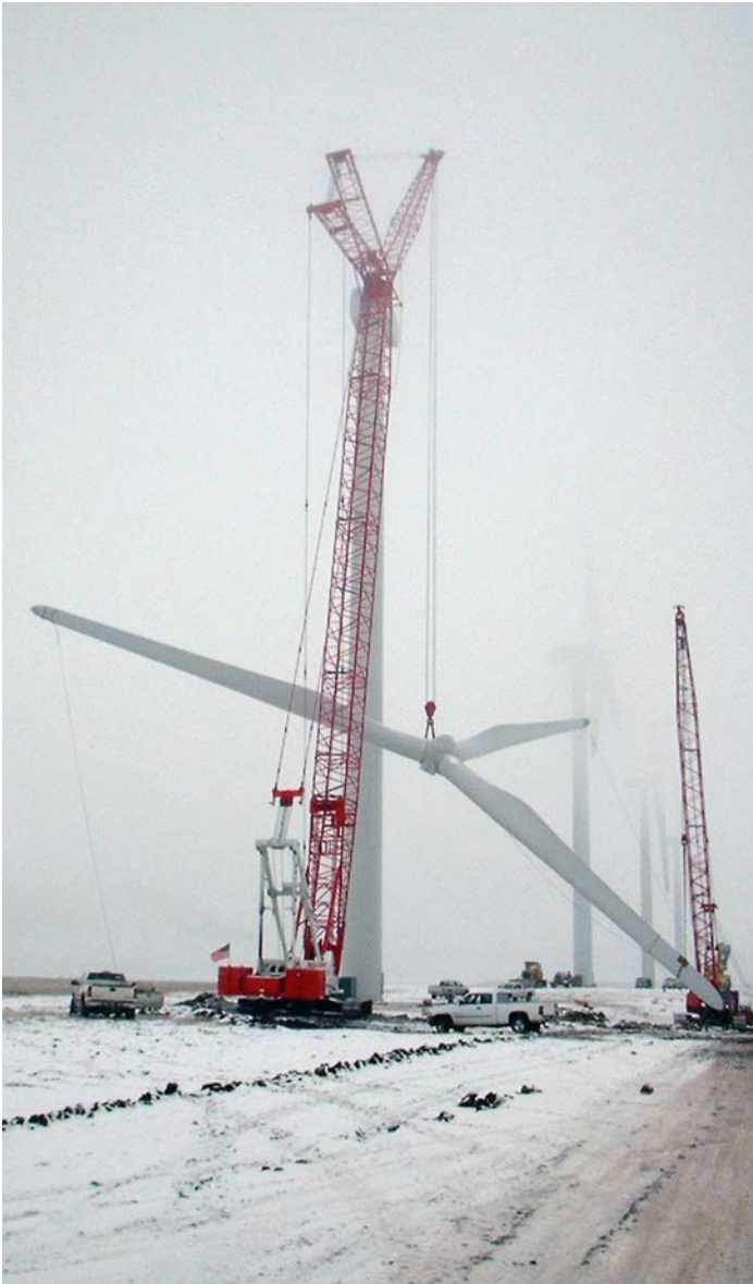
Small and large wind generation projects can benefit from the U.S. Department of Agriculture's Rural Energy for America Program Renewable Energy Systems & Energy Efficiency Improvement Loans. Photo from NREL, 11919
