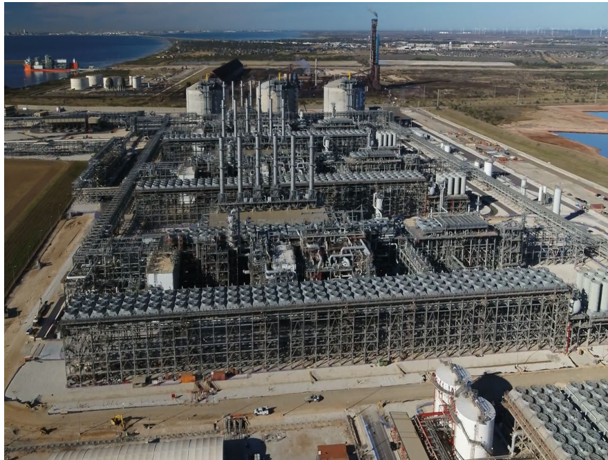
Overview CCL Stage 1 and 2 with LNG Tanks
