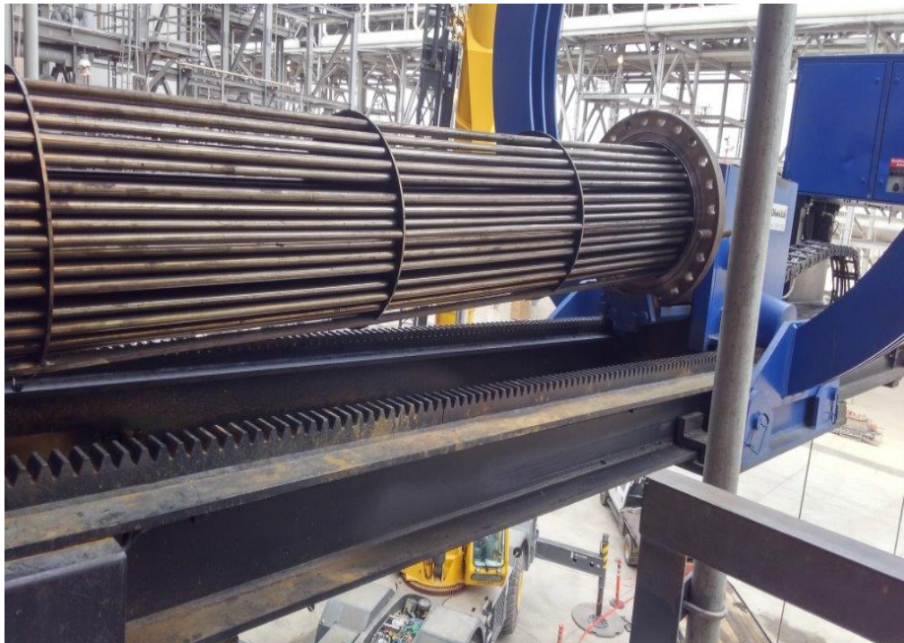
Ohmstede heat exchanger inspection
