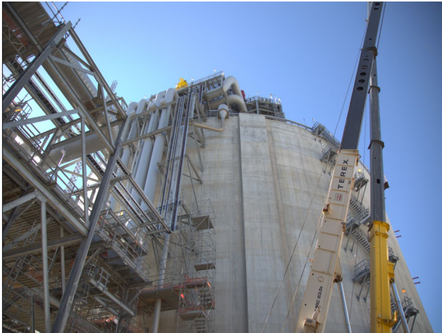
LNG Tank B - Overview of waterfall piping insulation
