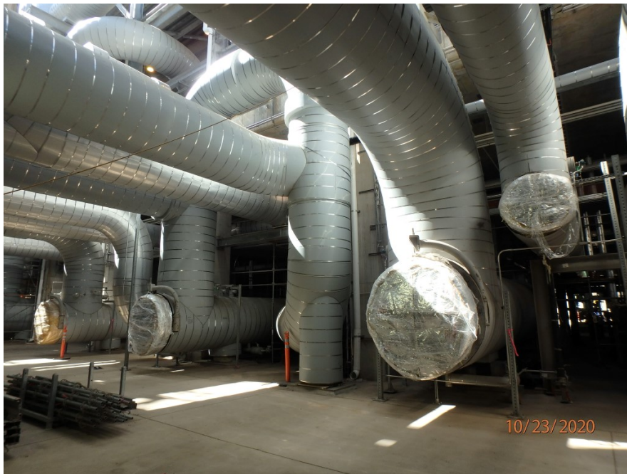
Alley way piping insulation with strainers leave-out
