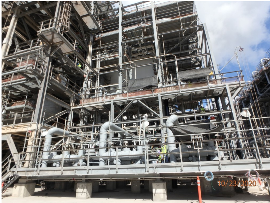
Heavies removal pumps installed
