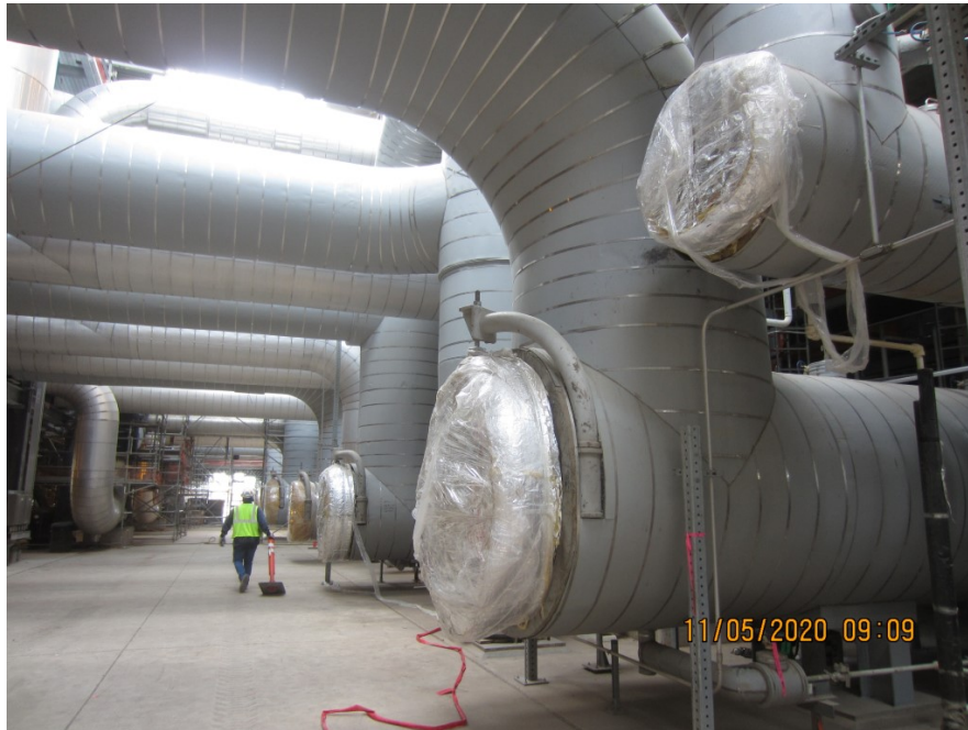
Train 3 - alley way piping insulation
