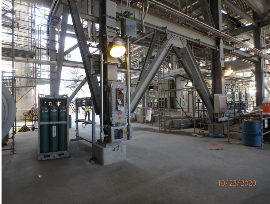
Analyzer shelter in service
