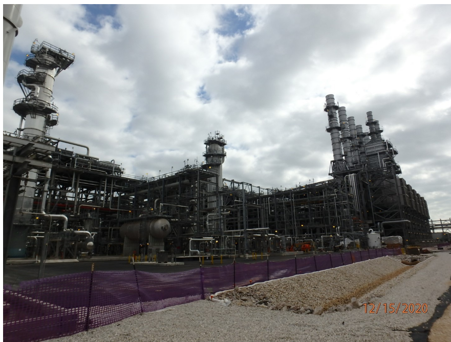
Train 3 in purple fenced ready for LNG production
