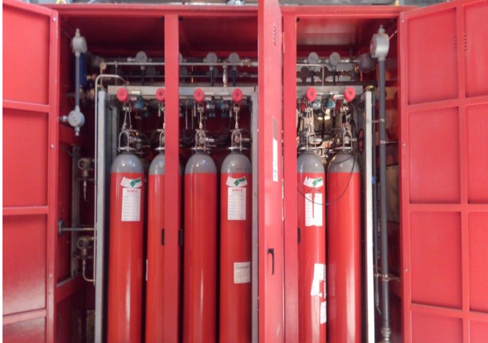
Refilling of CO2 bottles after dumb test on 1511 Compressor
