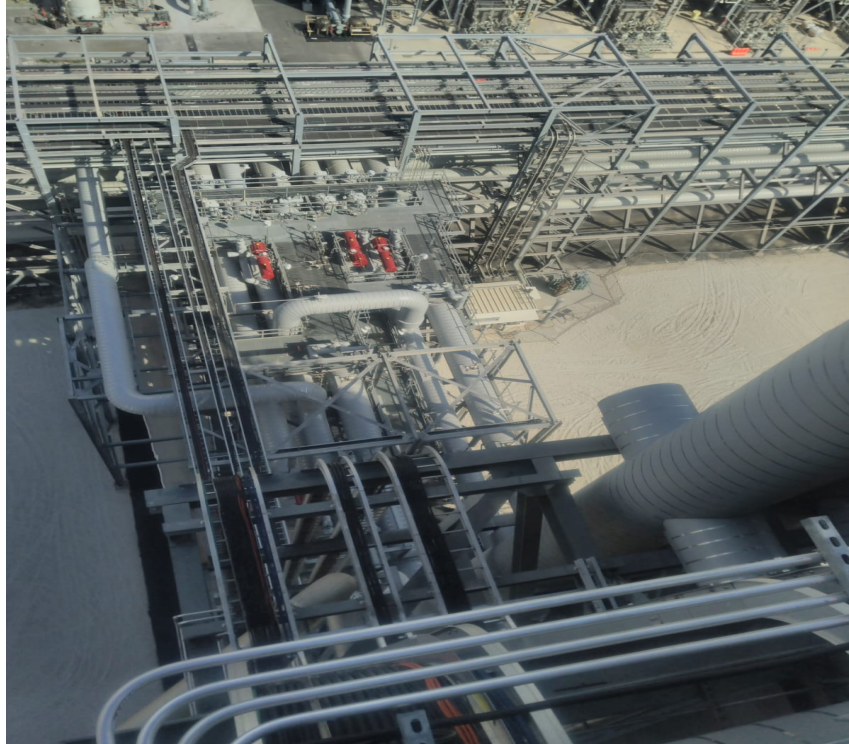
OSBL finger rack overview
