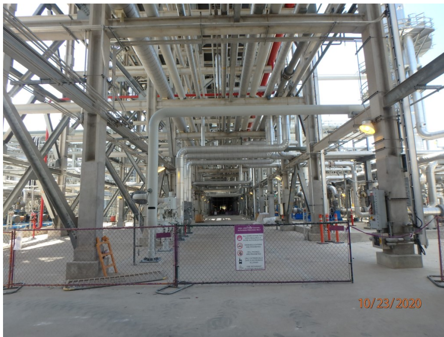
Purple fenced area for commissioning
