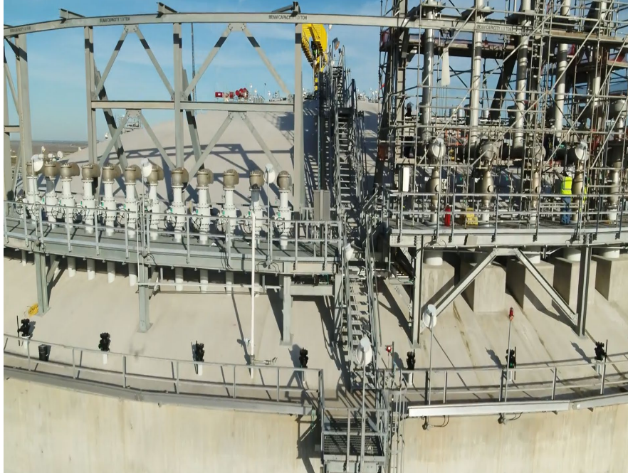
LNG Tank B - Vacuum breaker and valve platform
