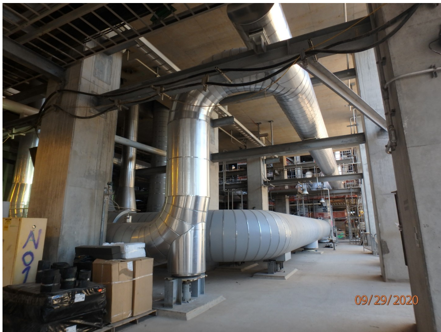
Methane compressor piping insulation
