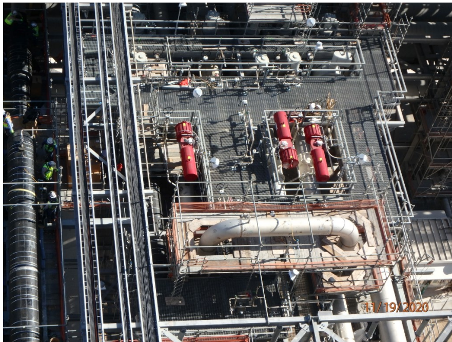
OSBL pipe rack - jump over and rundown piping insulation
