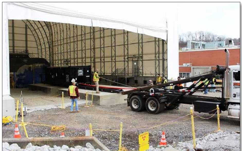
Workers built a multi-story temporary building to shield active-research areas of ORNL from demolition activities at two remaining hot cell structures. An intermodal rail system assists in efficient loading of debris for removal and disposition.
