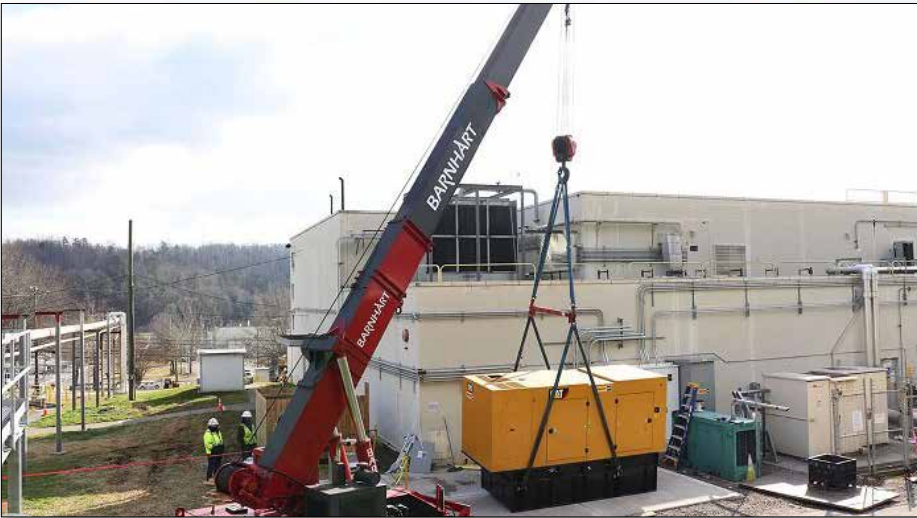
Workers install a backup diesel generator at Building 2026. If there is a loss of power, it can produce enough power to maintain operation of equipment necessary to process uranium-233 at Oak Ridge.
