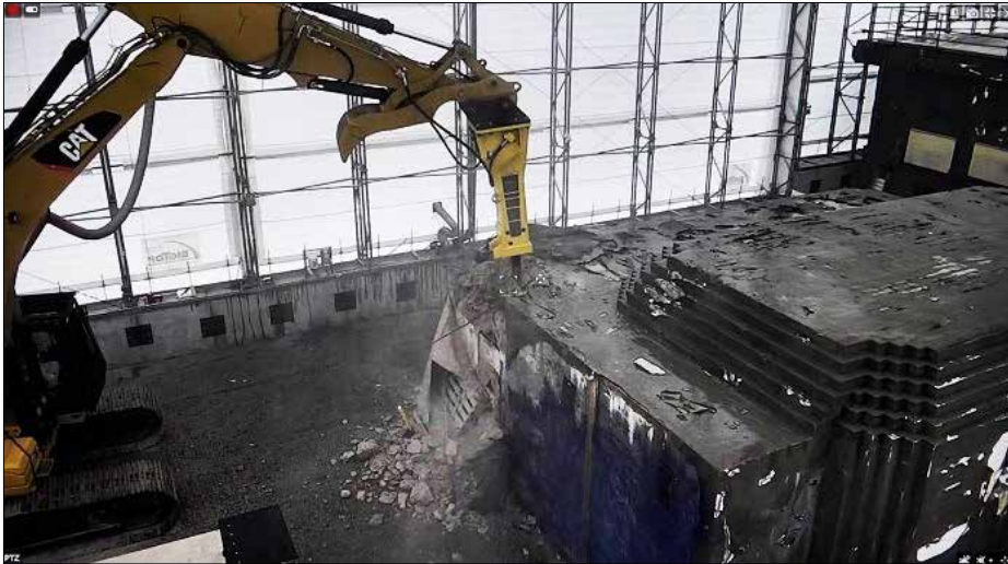
A view of the demolition of a hot cell inside a protective cover at the former Radioisotope Development Lab at ORNL.
