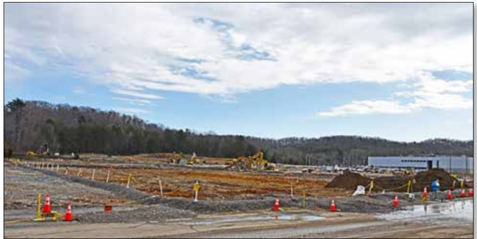
A view of the site where crews removed the building slab for the Centrifuge Complex.
