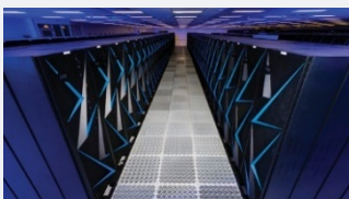
Sierra supercomputer at Lawrence Livermore National Laboratory in California
