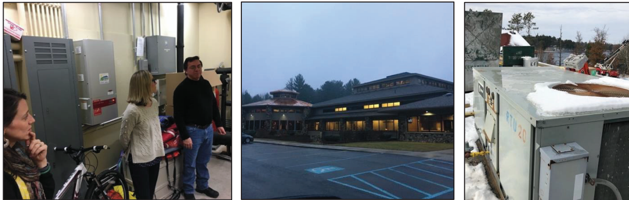
Figure 9: Photos of the Natural Resource utility room (left), the Dental Clinic (center), and an HVAC system (right) taken in December 2017 (top) and November 2018 (bottom). Photo credits: Sascha Petersen and Ellu Nasser.
