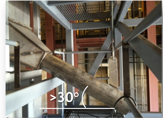
Pipe from particle elevator to top hopper
