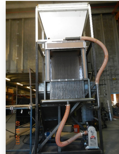
Pump and nozzles to produce air curtain across aperture
