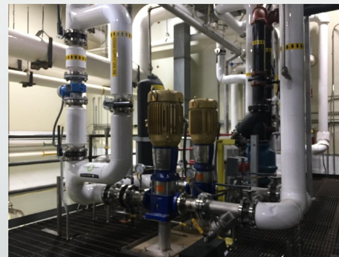
Heat Recovery Pumps and Heat Exchangers
