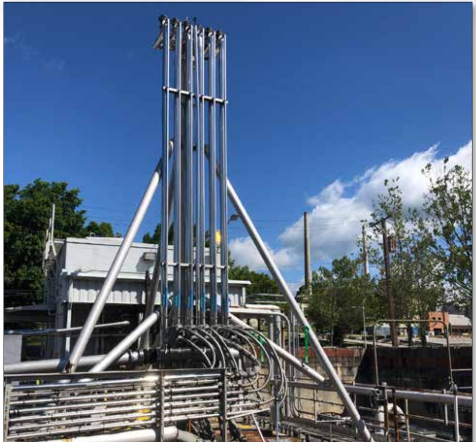
OREM continued progress on cleanup work at ORNL's Liquid Low-Level Waste System during limited operations. The system's barometric projection tower needs to be removed.
