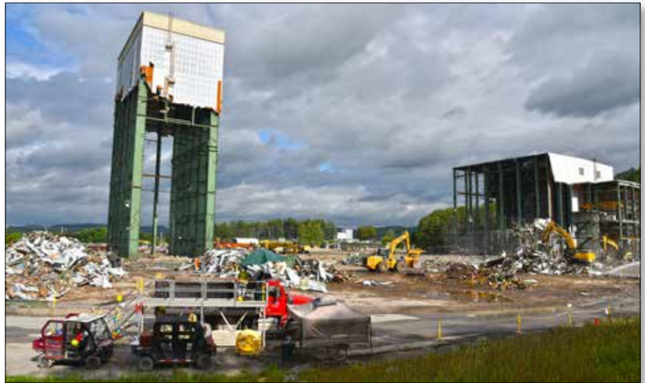
Crews are working to take down the final two facilities at ETTP's Centrifuge Complex. The K-1220 tower, left, was the tallest structure remaining on site before workers demolished it in June.
