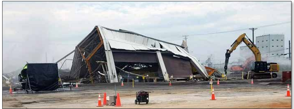
Oak Ridge crews spent several months completing deactivation work to prepare the K-1423 Toll Enrichment Facility for demolition.
