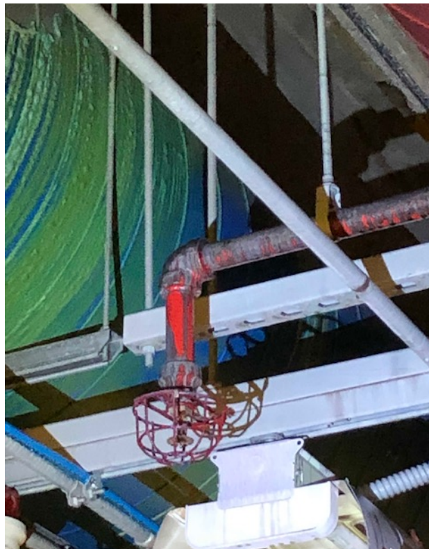
Figure 7. Sulfuric Acid Coating the Sprinkler Head
