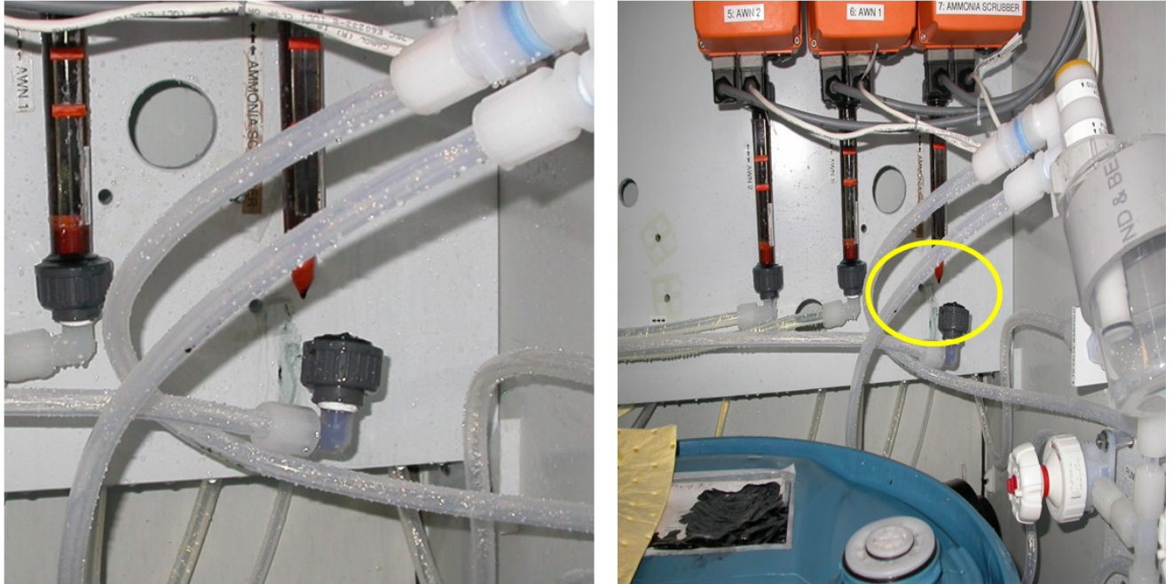
Figure 16. Failed Rotameter in the AWN Cabinet
