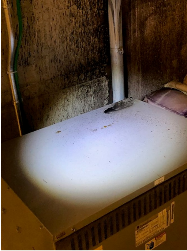
Figure 10. Sulfuric Acid on the Transformer
