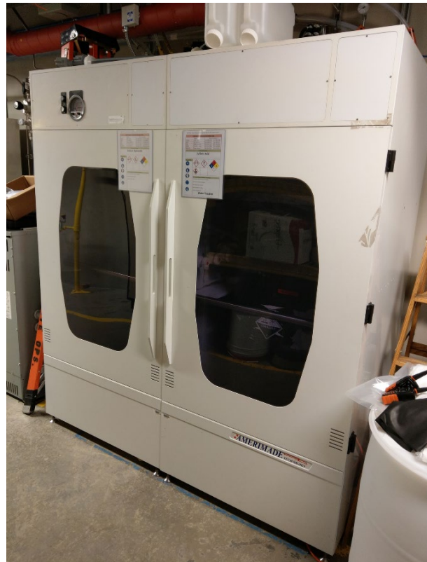
Figure 13. Automated Waste Neutralization System Chemical Delivery Cabinet
