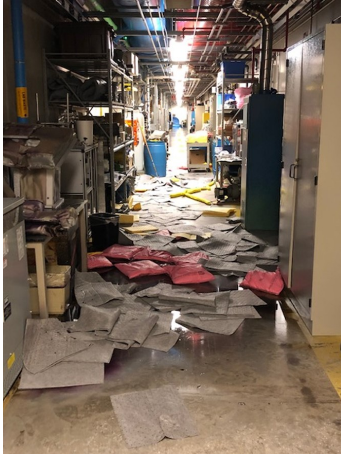
Figure 5. The first floor service corridor of S&TF after absorbent materials were applied to the acid that dripped through cracks in the concrete floor of the second floor.
