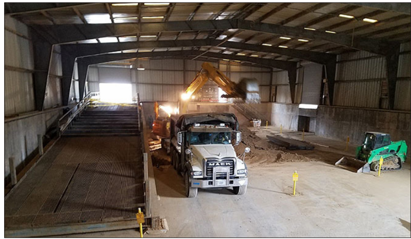
This photo shows workers nearing completion of the project to remove 4,071 cubic yards of soil that had been in storage in an Oak Ridge Site facility since 1989.
