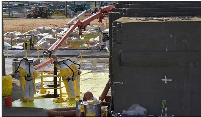
Oak Ridge workers grout a 47-foot-long underground transfer tunnel formerly used to load radioactive material into hot cells at Building 3026 at ORNL.
