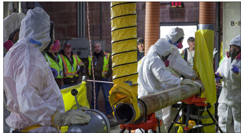
A crew tests a rotary machine with different attachments to remove crust and scale from the inside of the pipes of the Column Exchange equipment.
