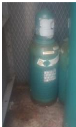
Figure 1: Small SF 6 cylinder last used 6 years prior, note rust creeping up from base of cylinder.
