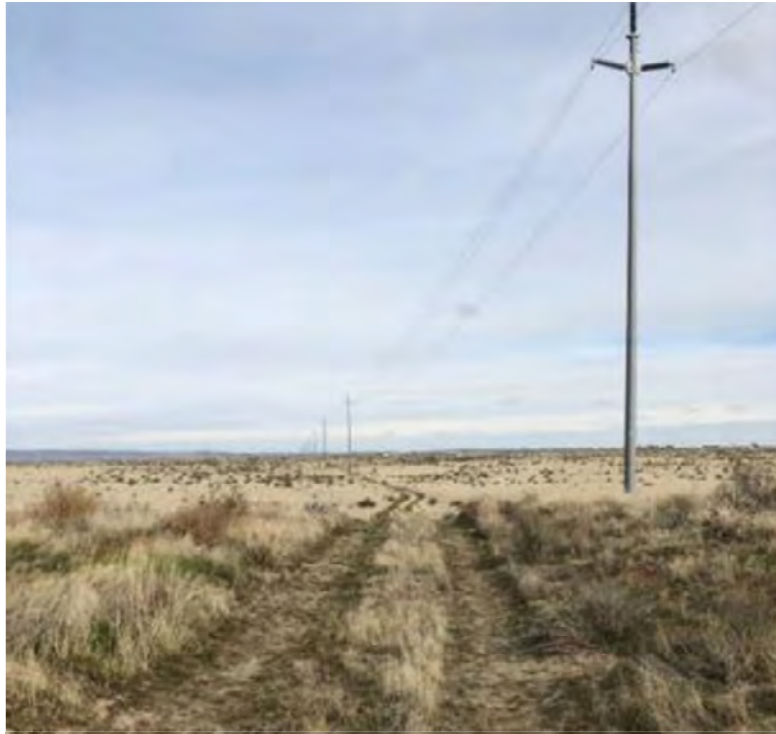
Figure 3-23. KOP-3 – White Bluffs – Single Pole Steel Structures Near Access Road Facing North
