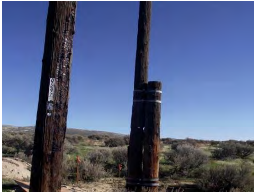
Figure 1-2. Deteriorated Pole with Fire Damage
