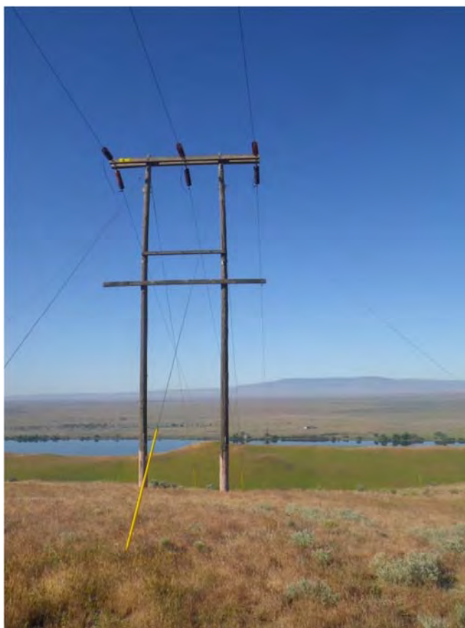
Figure 3-22. KOP-3 – Pole Structure from White Bluffs Facing South
