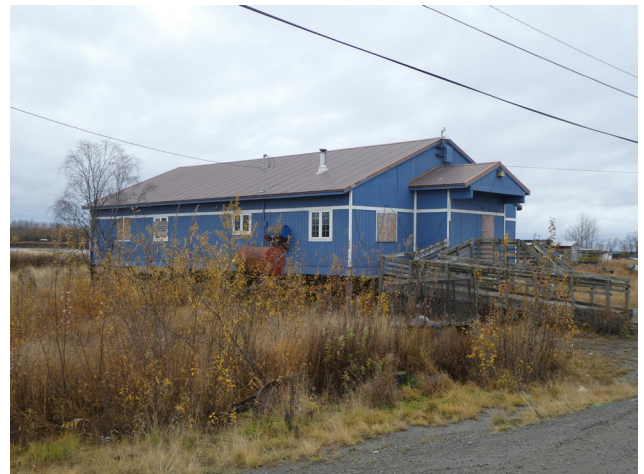
The Youth and Elder building needs rehabilitation so it will be safe to host more activities.
