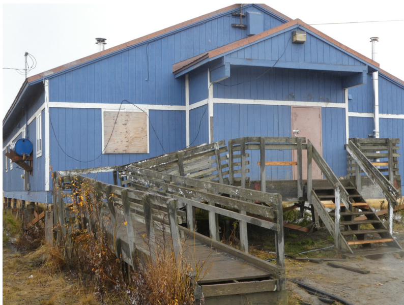
The top recommendation for the youth and elder building is to repair the failing foundation; this should be addressed prior to energy efficiency upgrades.
