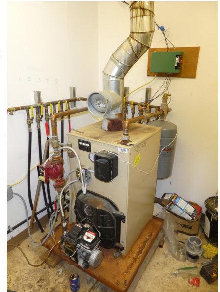
The boiler for the police station should be turned off during the summer to reduce energy costs.
