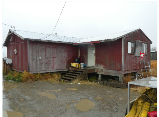
The jail is in poor condition and has no plumbing or exterior lighting.
