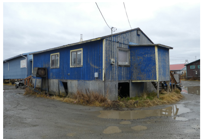
Despite comfort issues caused by poor lighting and cold drafts, the TANF building hosts around ten visitors each day.
