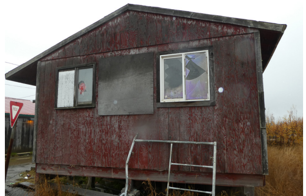
Cracked windows should be replaced when possible. This increases safety and comfort and decreases energy use.
