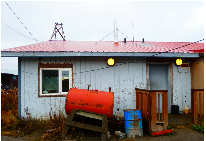
Like many tribal buildings in Akiachak, the police station has issues with malfunctioning thermostats and zone valves in its heating system.
