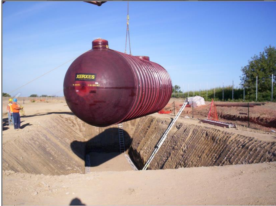
Figure 2-2. Installation of an Underground Storage Tank. Photo Source: Oscar W. Larson Co., Clarkston, MI.
