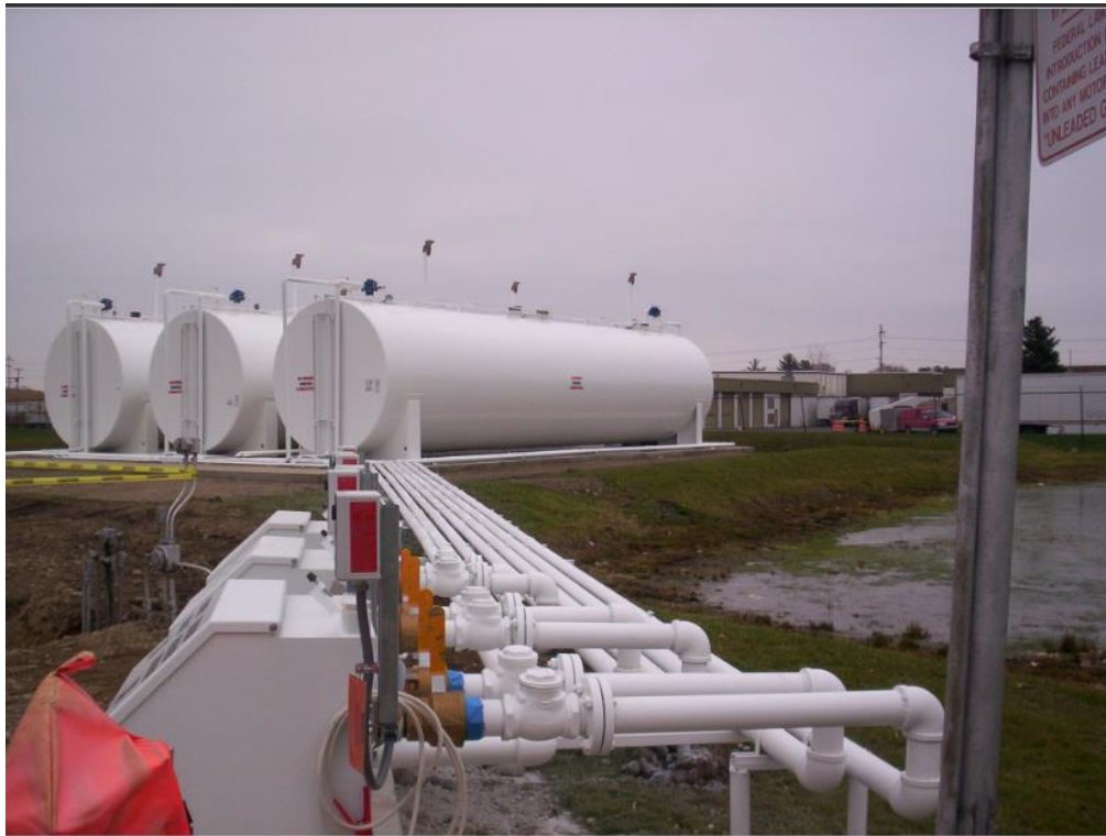
Figure 3-1. Fuel Supply Terminal. Photo Source: Oscar W. Larson Co., Clarkston, MI
