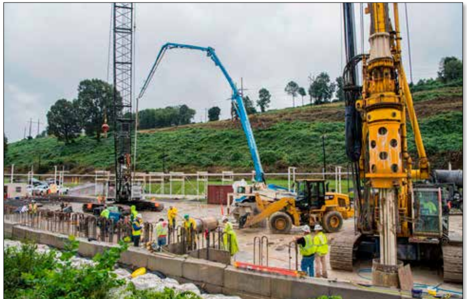
Building crews constructed two secant pile retaining walls to retain soils, control water seepage, and provide a deep, secure foundation for the water intake structure.
