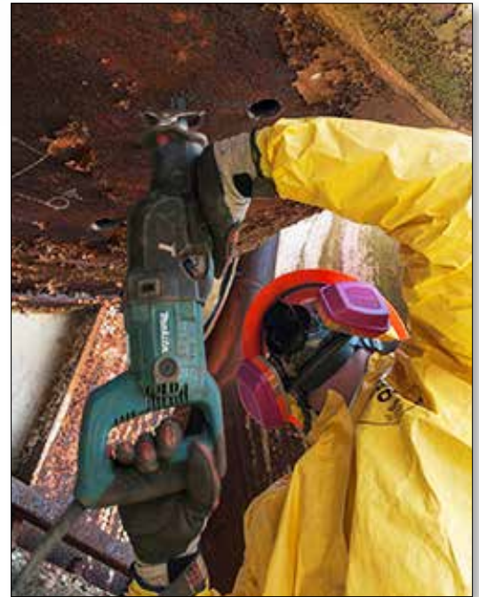
Crews drained mercury from the West Column Exchange pipes and equipment before demolition.
