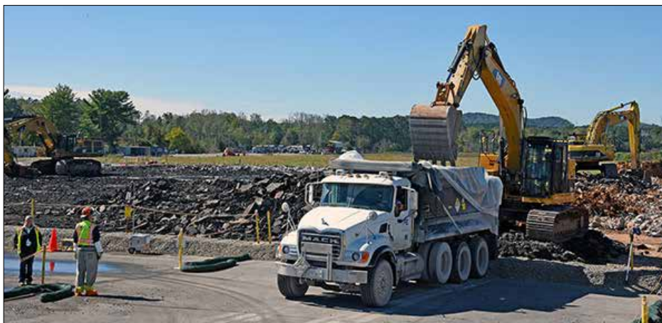
After crews finish removing the K-29 Building foundation slab in 2019, the Oak Ridge Office of EM will be set to transfer the area for industrial redevelopment.
