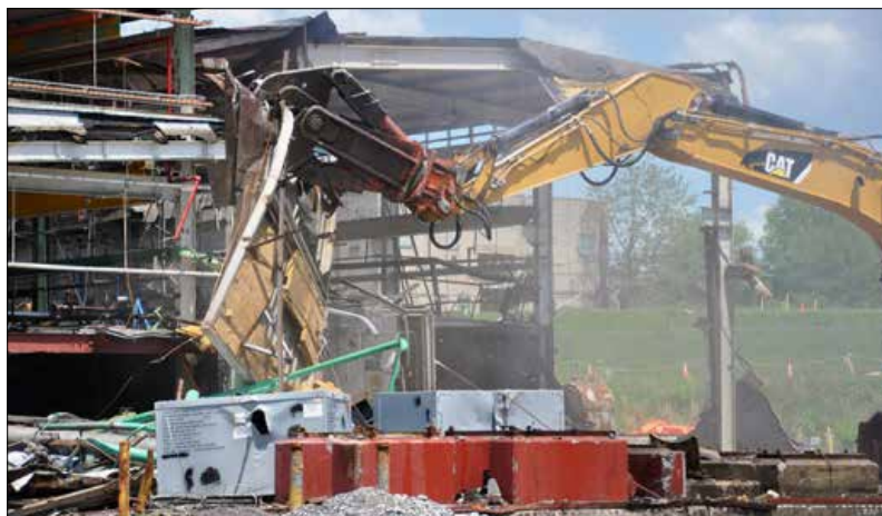
Crews began tearing down Building K-633 in May and completed the project in June.
