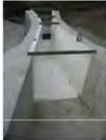
SSFL Area IV Outfall 5 bottom of drain into Brandeis-Bardin
