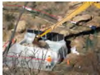
Contamination in drainage above Brandeis-Bardin dug out in 2007
