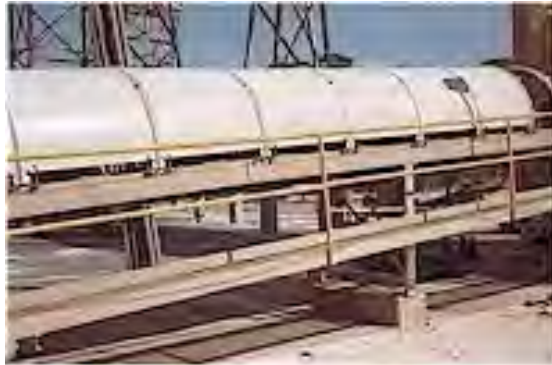
covered conveyor system
