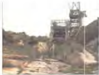
COCA Test Area in 2007 is in decrepit condition with lead paint covering the structure and massive amounts of TOE and perchlorate saturated into the dirt and groundwater around the stand which would remain if the decaying behemoth were "saved" resulting in no cleanup.
