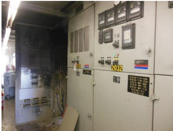
2015 LANL Electrical Arc
