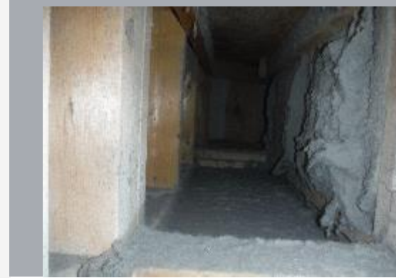
RETURN AIR PLATFORM
