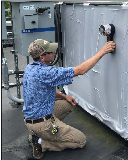
RTU Condenser Fouling Fault
