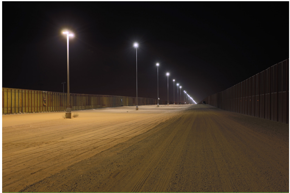
Yuma (AZ) Sector border lighting, showing the 40-foot pole height of the LED luminaires (on the first pole) and the 64-foot height of the incumbent QMH luminaires.
