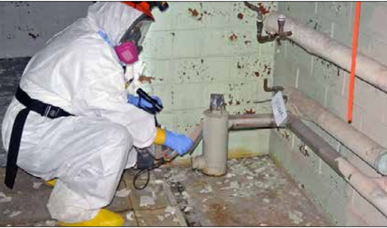
A technician surveys a pipe inside one of the buildings in the Biology Complex for contamination.
