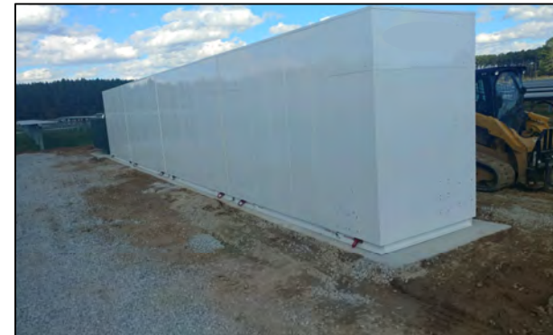
Redstone Arsenal, Alabama: 10 megawatt (MW) alternating current solar project with Army's first privately funded, commercially available battery storage solution
