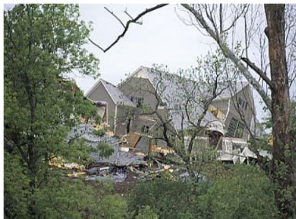
Source: (Kansas Geological Survey, 1999) Photo of Damage Caused by the 1995 Overland Park Landslide
