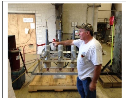
Figure 19. Testing Facility for Reclosers at CenterPoint.
