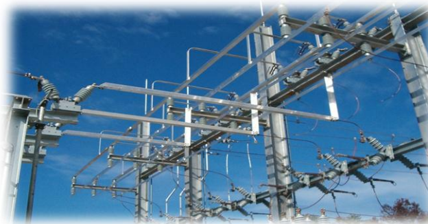
Figure 7. Example of GWP substation automation equipment.
