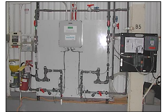
Advanced Controller at Fort Riley, KS
