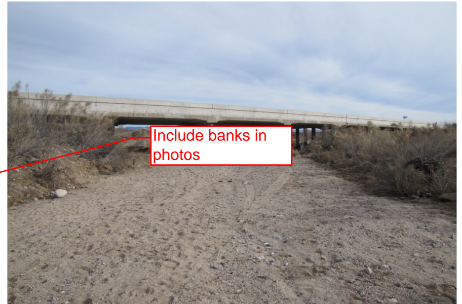
Gilson Wash, Photo 2. View downstream toward Gilson Wash Bridge from the west channel wash bed, facing northeast.
