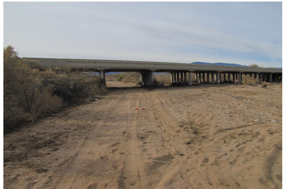
Gilson Wash, Photo 8. View upstream toward Gilson Wash Bridge from the wash bed, facing southwest.
